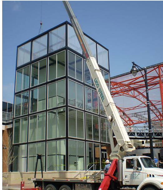
Figure 10. ETFE glazing for the KCPL Facades, Kansas City, US.
