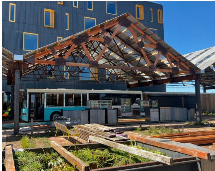
Figure 40. Under construction—Bobby's Bakehouse and the pie bus, resurrected from an old school bus and other materials on site Source: Stockland (2023)
