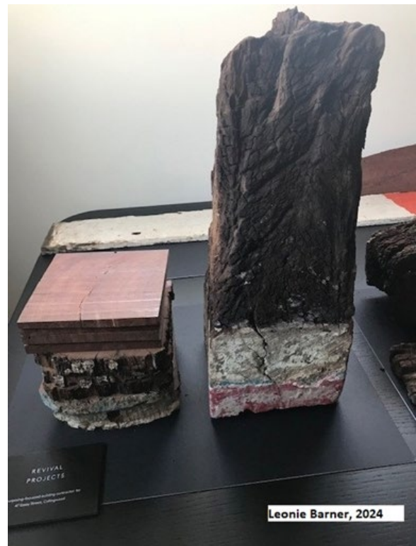
Example of partly rotten wooden load-bearing column. Left: Intact wood samples that were extracted from the load-bearing columns.*
