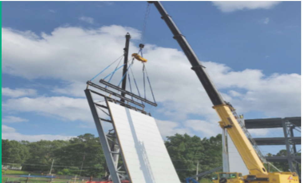
Figure 5: Installation of prefabricated wall modules with Verton's remote load control system and RBD/HALE Steel's Tilt Table
