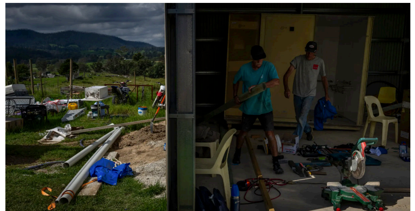
Figure 4: A bathroom pod being installed in a shed as a work-around for a disabled resident in a temporary accommodation pod, so they can shower while they wait for the rebuild. Image credit: The Guardian
